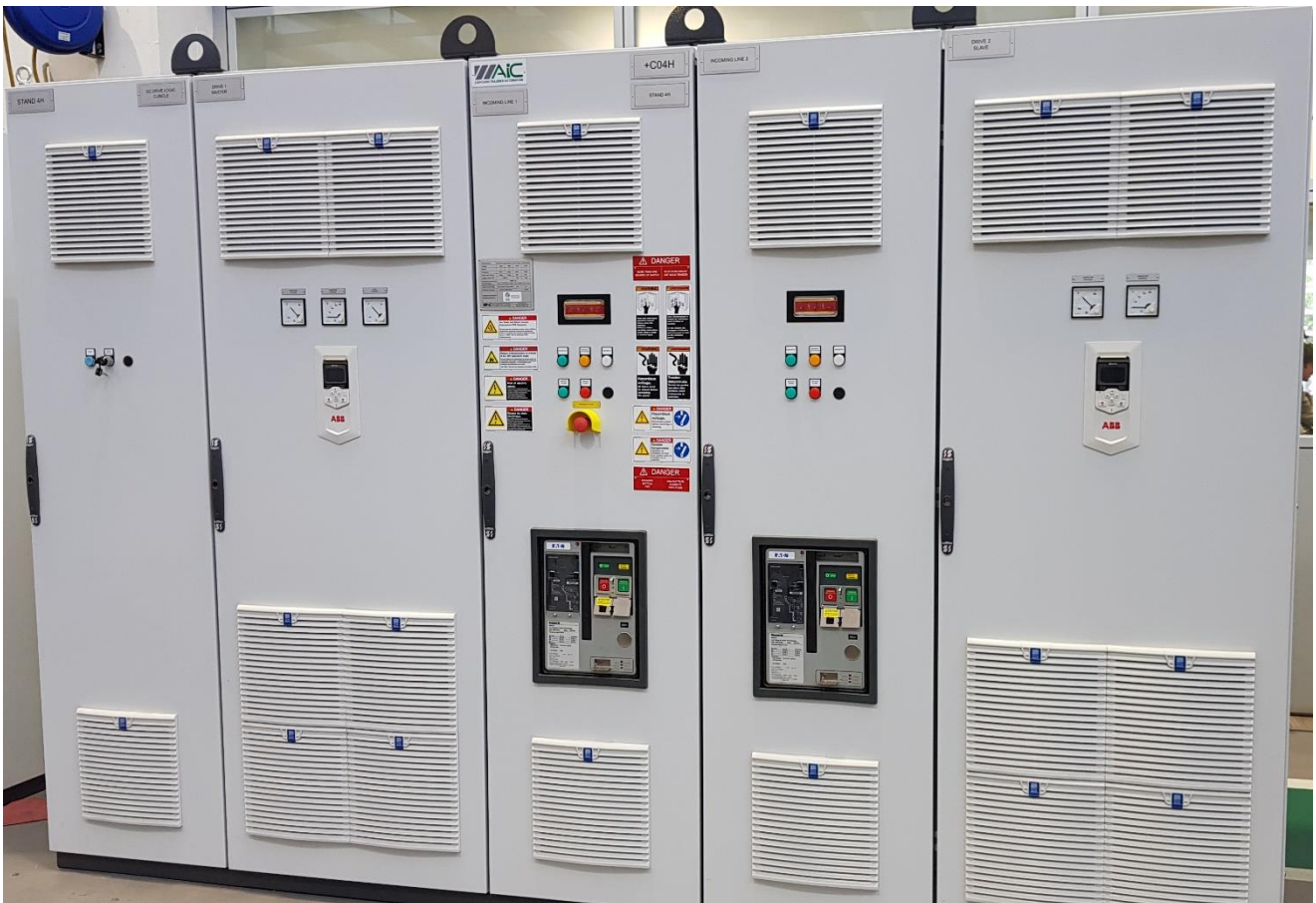
(one of recent stands drives installed at site)
