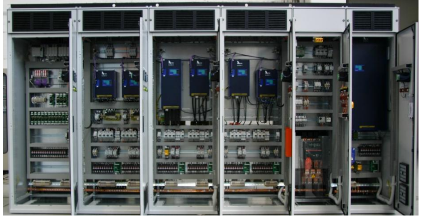
Fig. 18 – New auxiliary DC Drives panel
