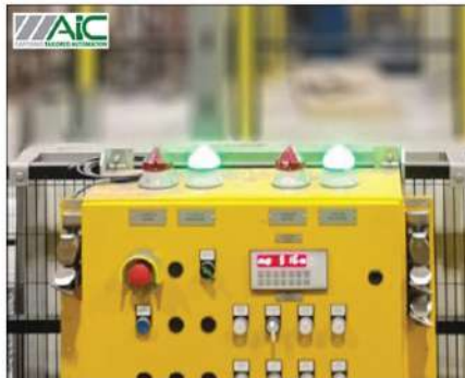
Fig 24 Safety boxes with alarms
